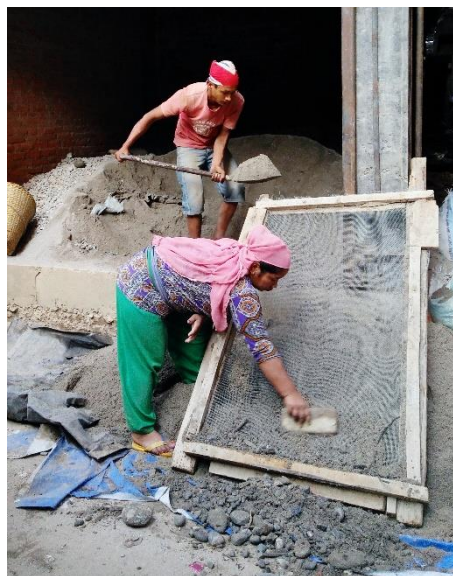
Workers at the Manohar Construction site where our team conducted some of their field studies in Kathmandu, Nepal
